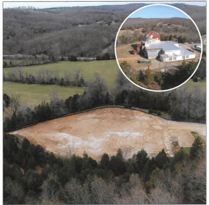
The SEFOR decommissioning project began in 2017, and was completed with the dismantlement of all above-grade structures; cleanout and removal of all systems, structures, and components from below grade; and the removal of the reactor and ancillary equipment.
